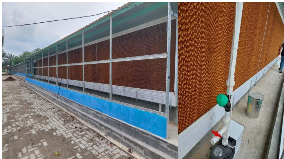
gambar lampiran 7 system colling pad
