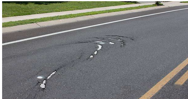
Gambar 2.16 Patah Slip ( Slippage Cracking ) Sumber : Bina marga no.03/MN/B/1983
