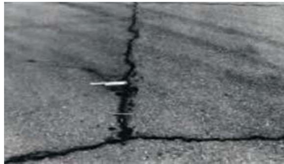
Gambar 2.8 Retak Sambung ( Joint Refle Cracking ) Sumber : Bina marga no.03/MN/B/1983
