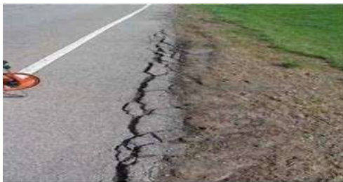
Gambar 2.7 Retak Samping jalan ( Edge Cracking ) Sumber : Bina marga no.03/MN/B/1983
