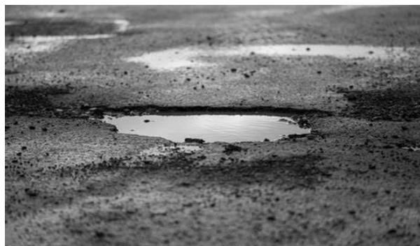
Gambar 2.13 Lubang ( Pothole ) Sumber : Bina marga no.03/MN/B/1983
