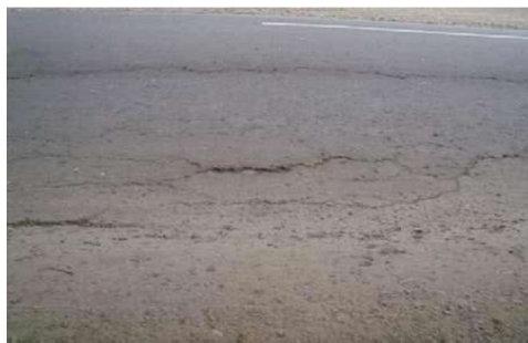
Gambar 2.4 Cekungan ( Bump and Sags ) Sumber : Bina marga No.03/MN/B/1983
