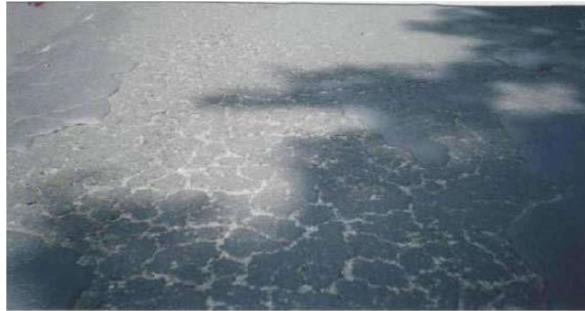
Gambar 2.18 Pelepasan Butir ( Weathering/Raveling ) Sumber : Bina marga no.03/MN/B/1983
