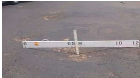
Gambar 2.6 Amblas ( Depression ) Sumber : Bina marga no.03/MN/B/1983
