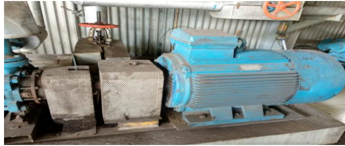
Gambar 2.13 Feed water pump
