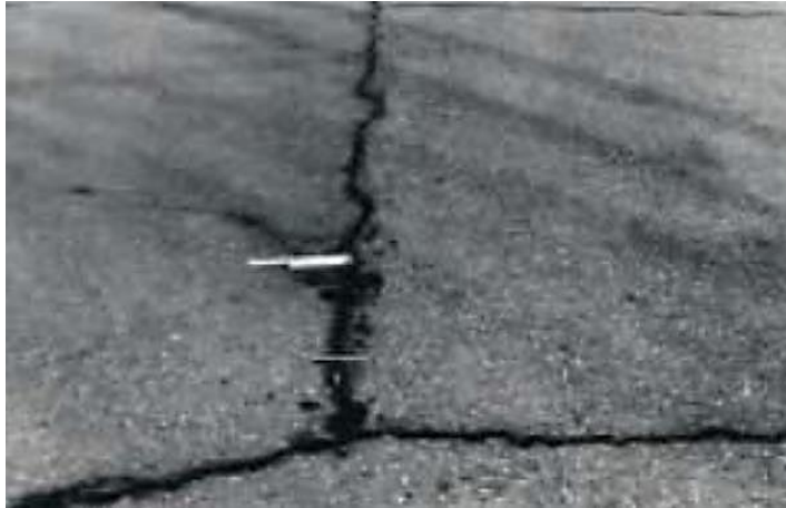
Gambar 2.7 Contoh Kerusakan Sambung ( Joint Reflection Cracking )
