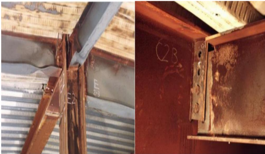
Gambar 2.1 Kegagalan Sambungan Baja Sumber: ( https://id.pinterest.com/pin/412360909624256420 )
