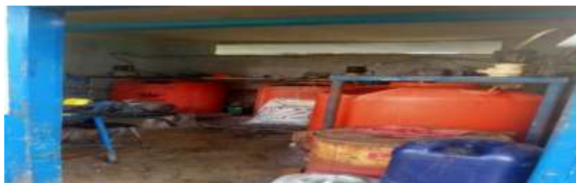
Gambar 2.2 Tangki penambahan bahan chemical
