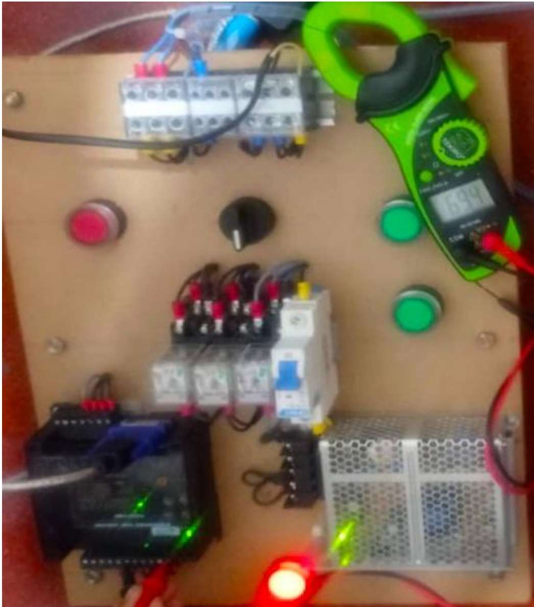
i. Pengujian selector switch mode off
